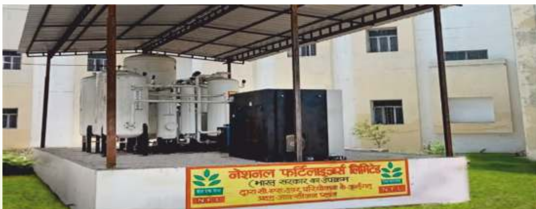
The company installed & commissioned 04 nos. Medical Oxygen Generator Plants at Bhopal, Lucknow, Gorakhpur & Indore to strengthen the Covid Care facilities
